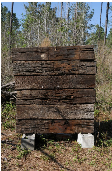
Figure 1. Space the left and right cinder blocks according to the width of the backstop you are constructing.
